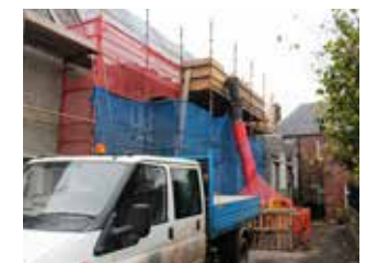
Access scaffold erected to allow high level roof repairs to principal elevation.
